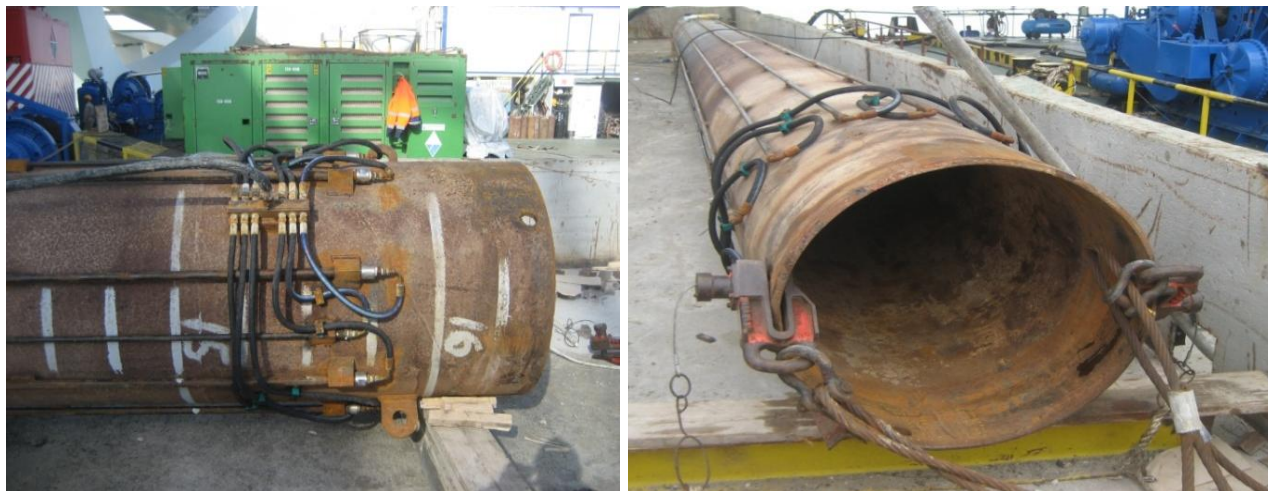
Figure 9. Distribution Lines on top of Casing Pile.
