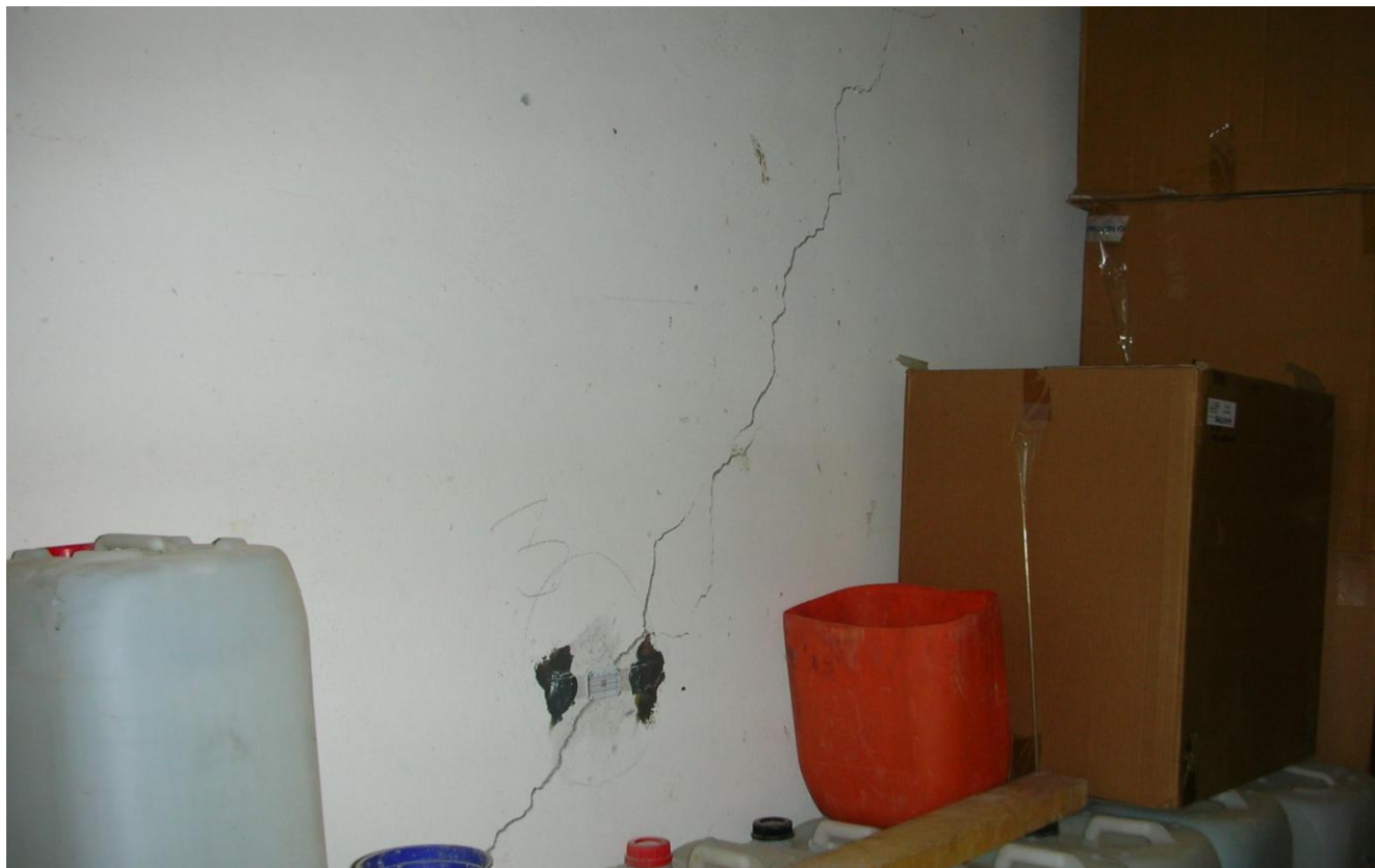
Figure 2. Wall damage inside the warehouse.
