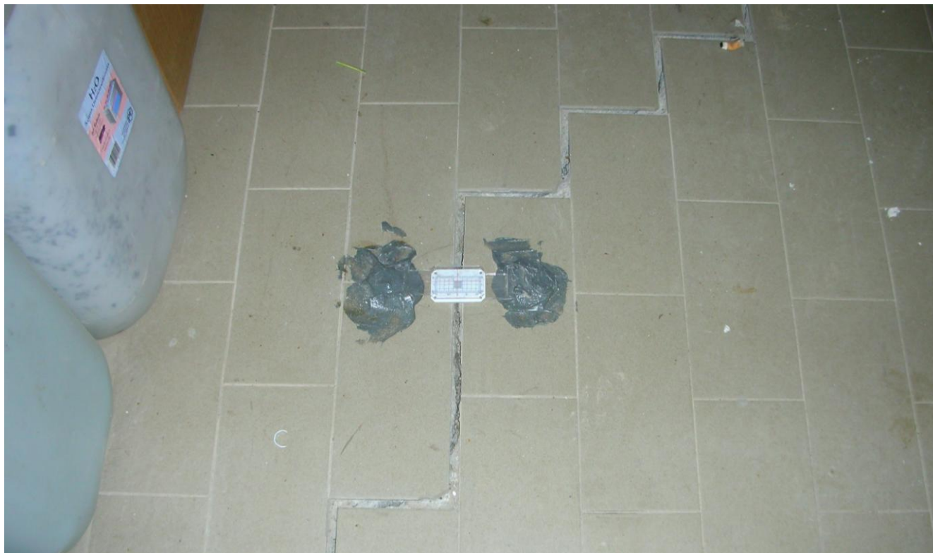
Figure 3. Floor damage inside the warehouse.
