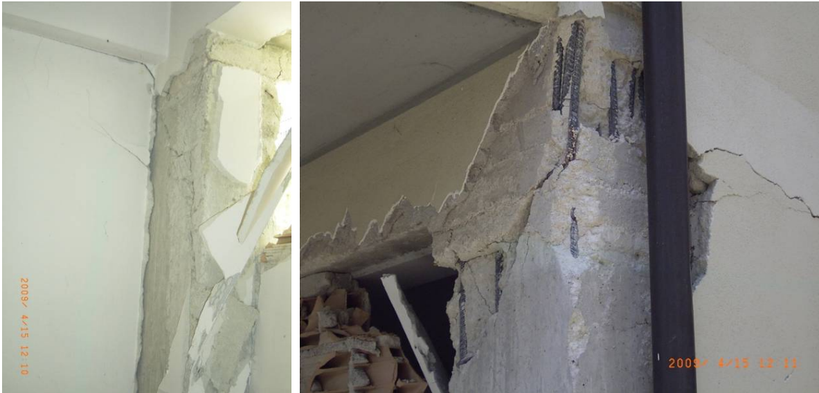
Two photographs showing the aftermath of an earthquake. The left photo shows a collapsed balcony with a metal railing and debris on the ground. The right photo shows a damaged brick wall and a collapsed metal railing.
