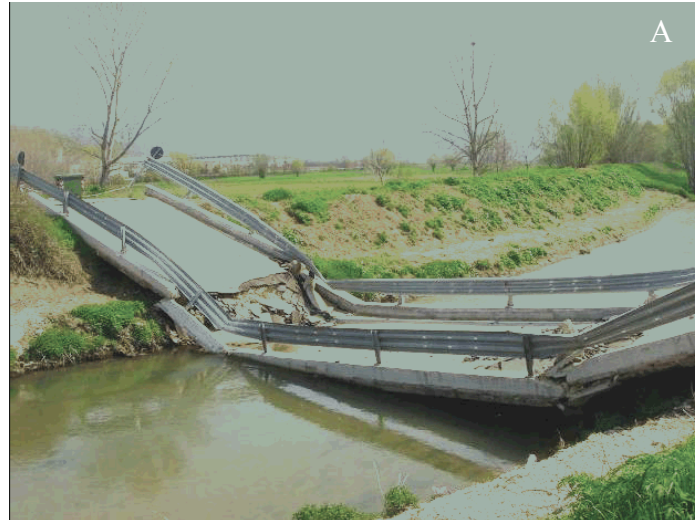
Figure 68. Onna. (A) Collapse (D5).
